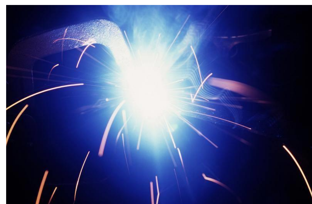
Figure: Bright light during welding
